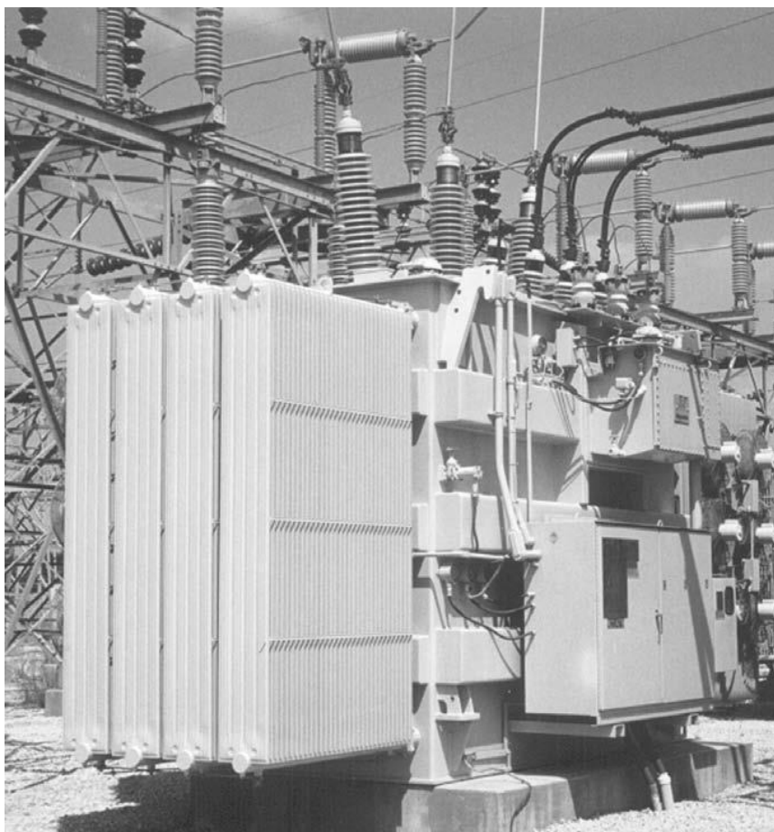
101-rasm. Taqsimlovchi kuch transformatori
