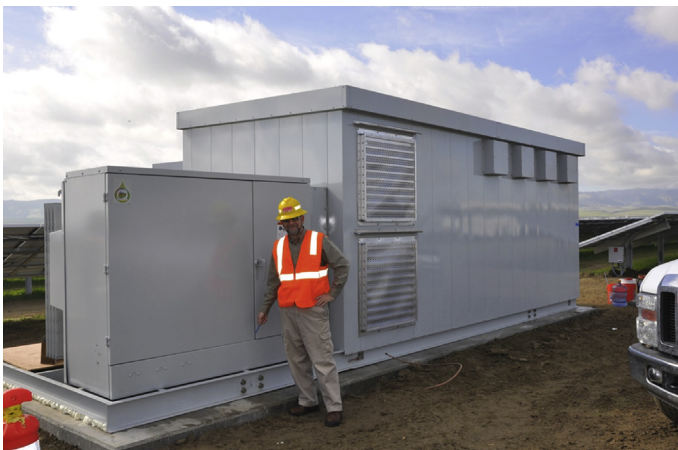
Figure 1.1 A typical electrical shelter.
