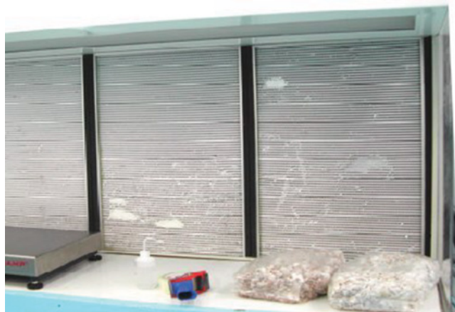
Figure 5.23 Damaged HEPA filters in need of replacement.
