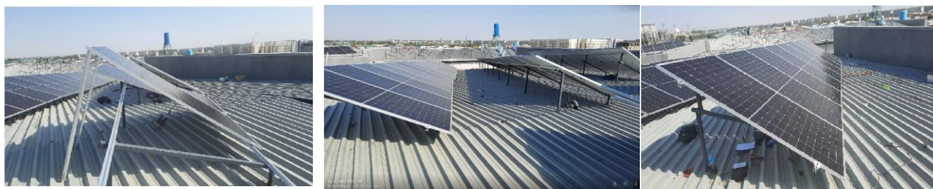
Figure 2. Measuring and setting PV module parameters in natural conditions
